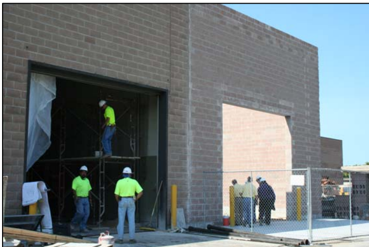
New spray booth work – demolition in existing maintenance garage to tie the bays together
